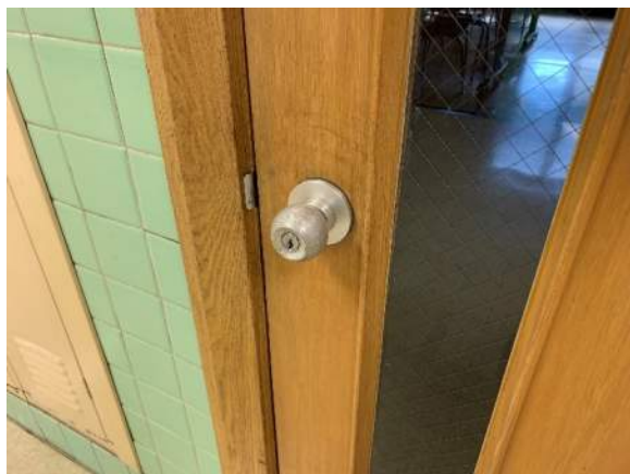
Photo A08 – Non-compliant Door Handle
