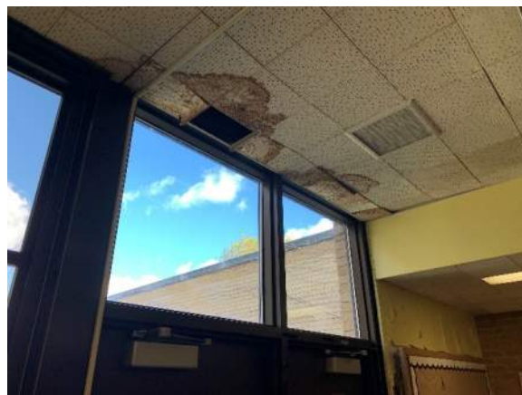
Photo A09 – Water Intrusion Damage
