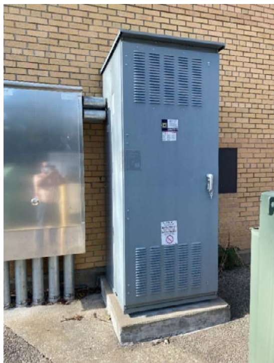
Photo E01 – Service Entry Switch
