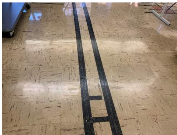
Photo A19 – Asbestos Floor Tile
