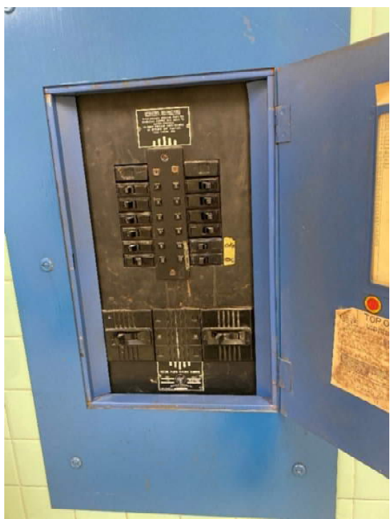
Photo E03 – Branch Circuit Boards
