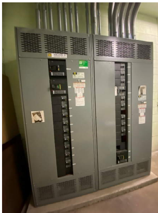
Photo E02 – Main Distribution Panel
